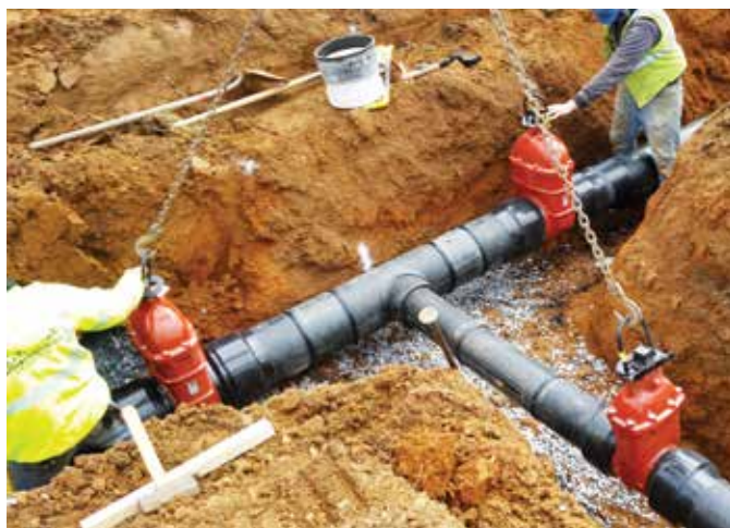
Shut-off valves and fire hydrants were heat fused into the HDPE pipeline to further ensure a leak-free, closed loop system
