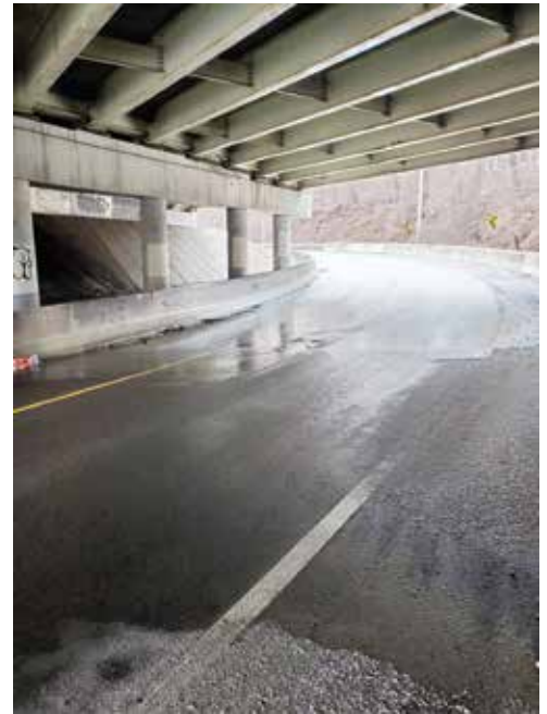
Figure 3. Water main breach was flowing onto the South Bound offramp to I-83, creating hazardous conditions
