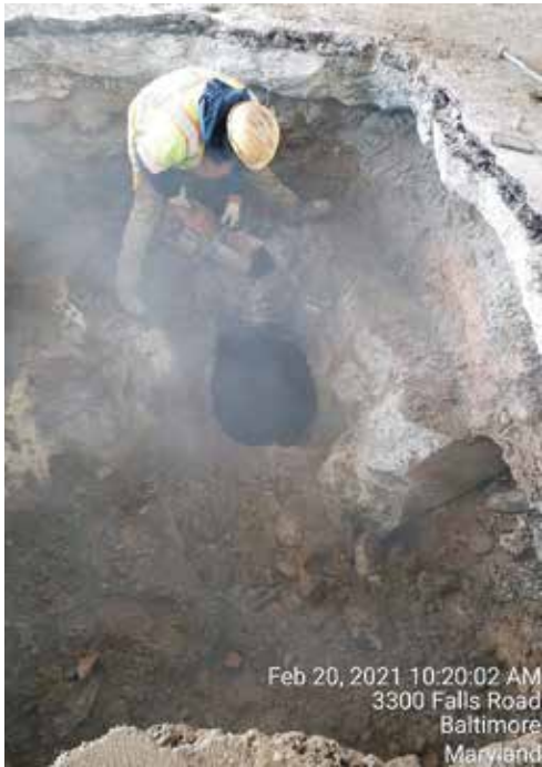
Figure 5. A two-foot hole was cut into the water main to inspect for further damage
