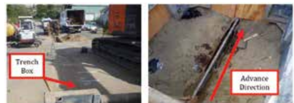
Figure 2 - Vermeer D36x50 Setup (Left); Drill Pipe Entering Existing 8-inch VCP in Trench Box (Right)
