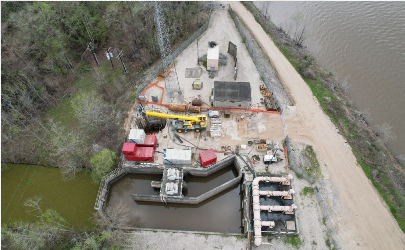
Figure 9. Photo of Shaft and Limited Working Area at the Existing Lawson Raw Water Pump Station
