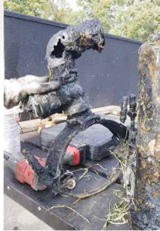
Figure 2: Broken Air Release Valve due to H 2 S Damage
