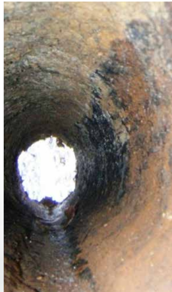
Figure 3: Pipe Invert Abrasion
