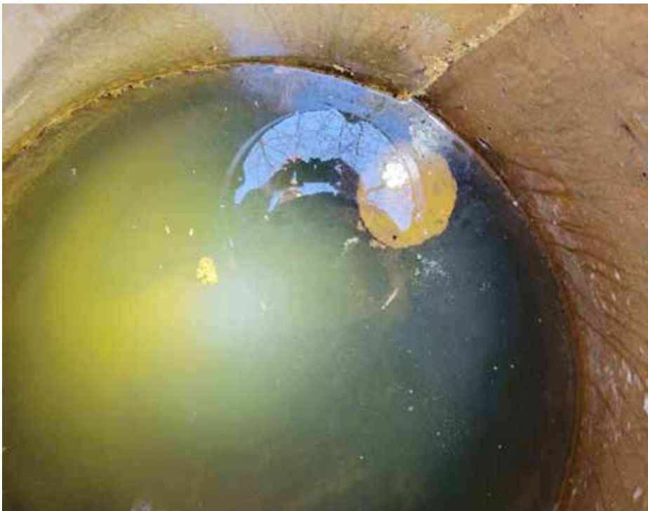
Figure 7: Submerged Air Release Valve
