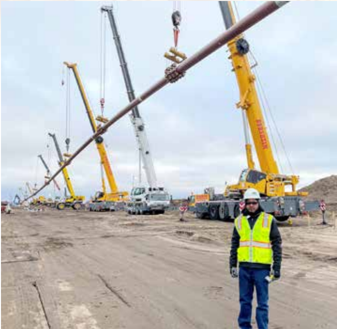
Kerby Primm on project site of record-long underground crossing Lake Sakakawea ND
