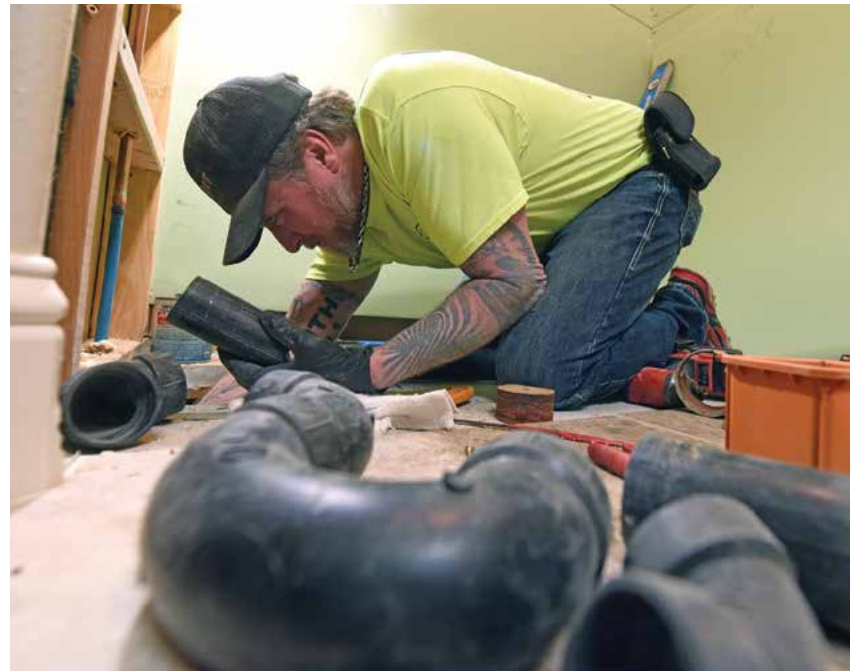
» J.D. cuts pipe during a shower installation. The company still takes on traditional plumbing work, but less so these days.
