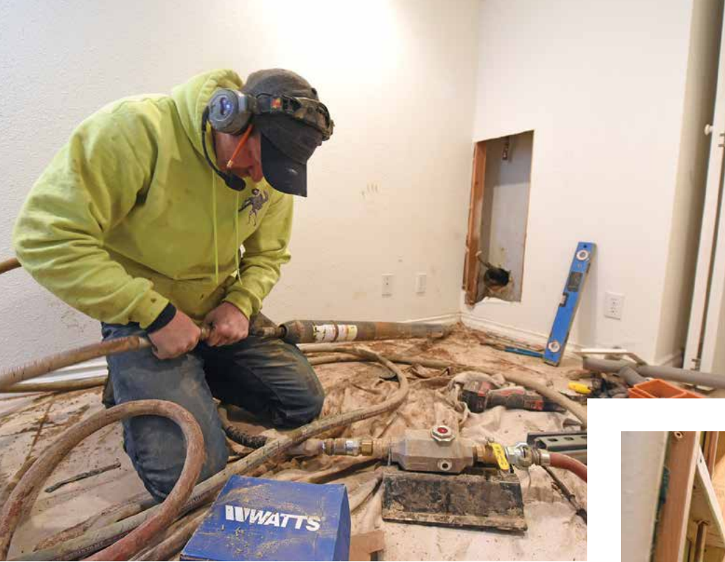
« Technician Zach Hall disconnects an air hose from a Vermeer pneumatic hole hammer.
