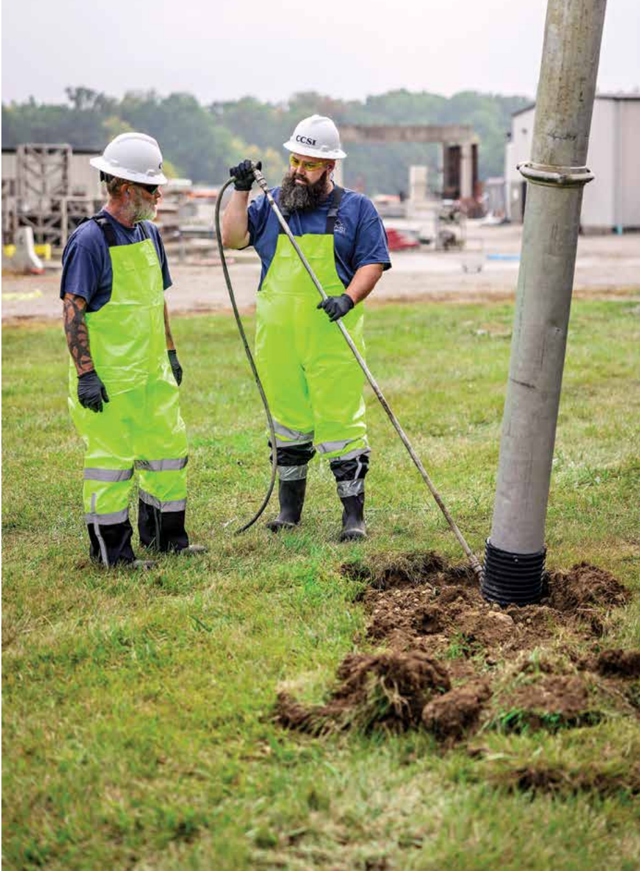
« Scott Oliver and Nick Mason work on a hydroexcavation job in Monroe, Ohio.
