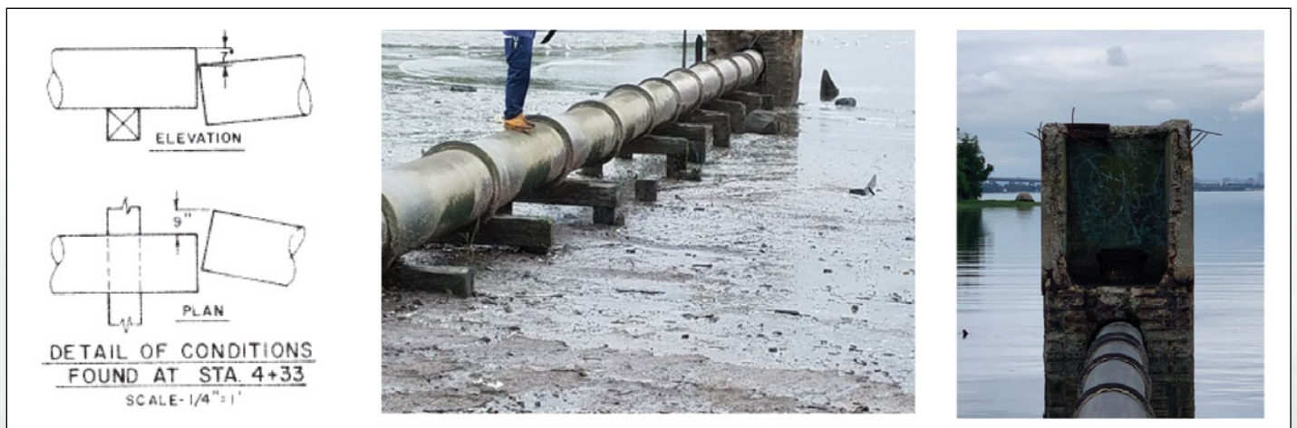
Figure 3. Damage to existing outfall and manholes
