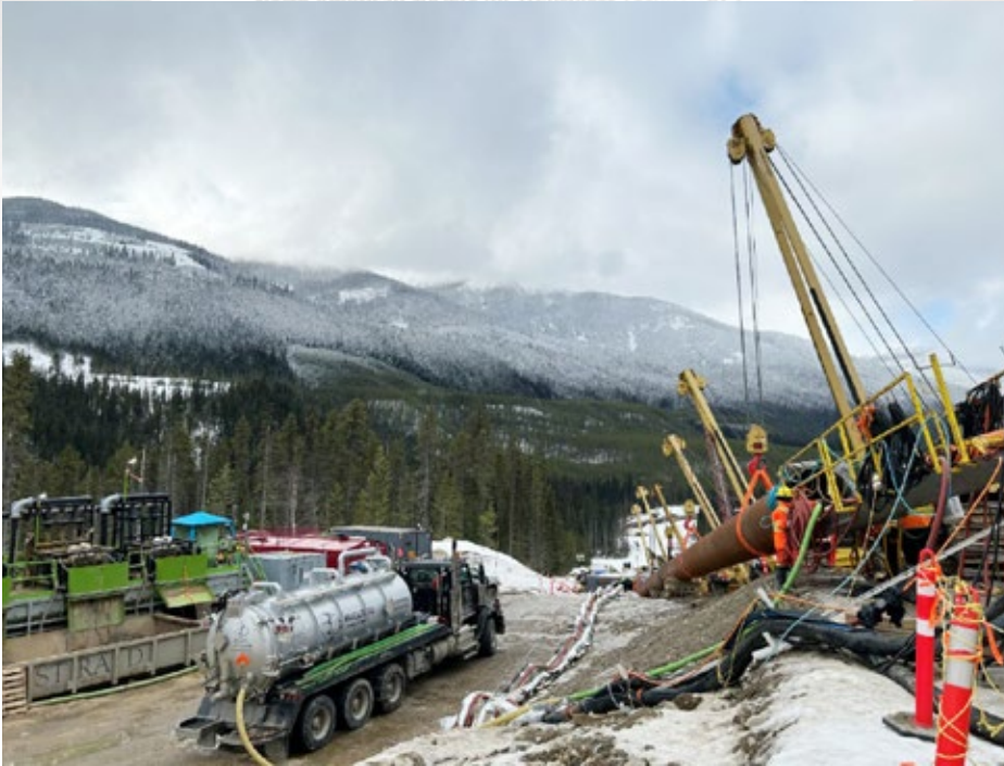
Figure 9. Albreda Triple Crossing Looking down from Launch to Reception
