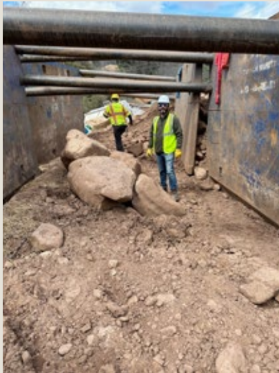
BEFORE: A worker stands next to boulders retrieved during excavation of the launch pit
