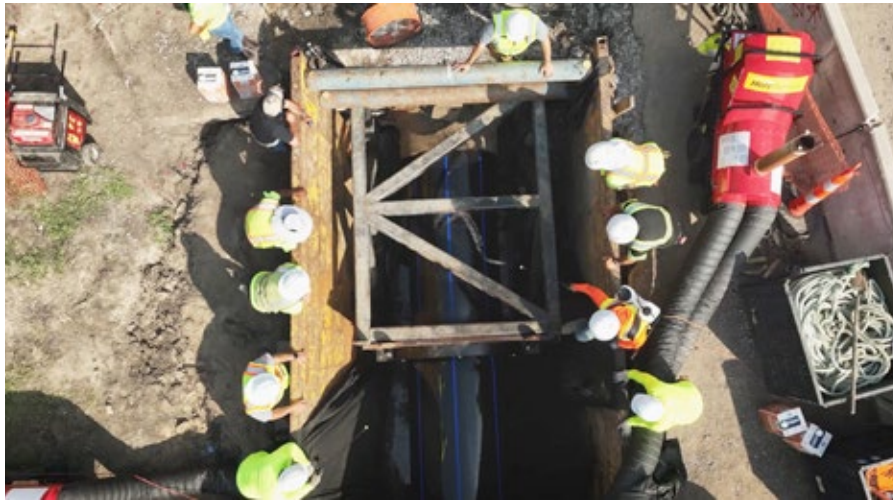
The CompressionFit method helped reduce overall project costs and minimize traffic disruption
