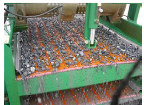
Figure 1 Coarse Screen on Microtunneling Slurry Separation Plant
