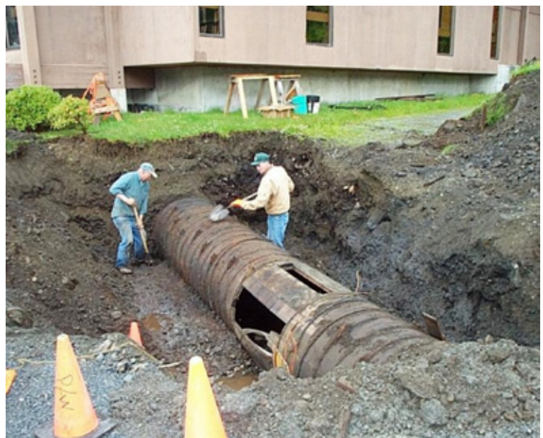
Figure 2. Exposing the Damaged Penstock Pipe in 2001, Note Library Proximity in the Background
