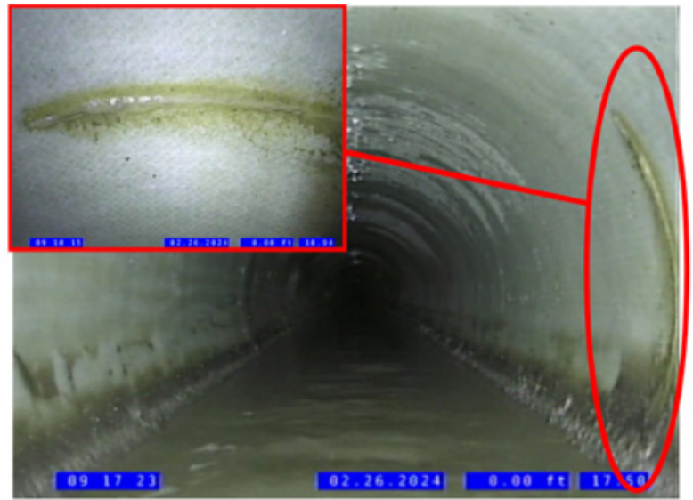
Figure 11. CCTV Inspection Footage of Pinholes in Cured Liner
