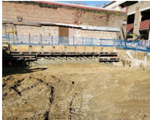
Figure 1: The Bressi Building, a historic structure requiring preservation during the Climate Pledge Arena construction
