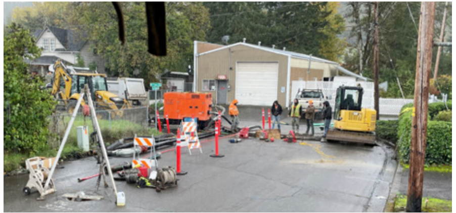
Figure 9. Sanitary Sewer Bypass Piping Entering Stormwater System
